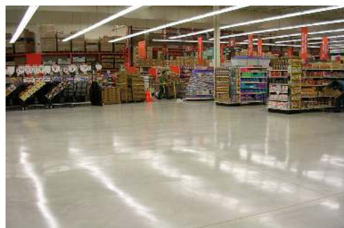
Typical steel trowel finished concrete with one coat of Durafloor HD and three coats of Durafloor HD-S.
